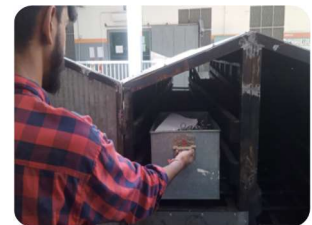
Install the mild steel bridge by replacing of using handcart. Travel distance reduced 60 m to 12 m
